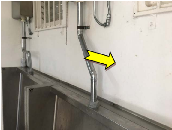
Photo 9. Interior, male toilets, walls – suspected lead-containing white upper paint systems.
