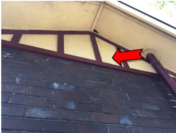
Photo 3. Exterior, ladies toilets, gable end – suspected asbestos-containing fibre cement sheeting.
