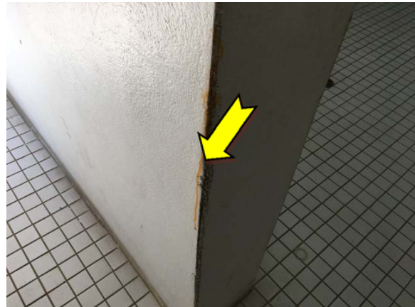
Photo 10. Interior, male toilets, walls – suspected lead-containing yellow lower paint systems.
