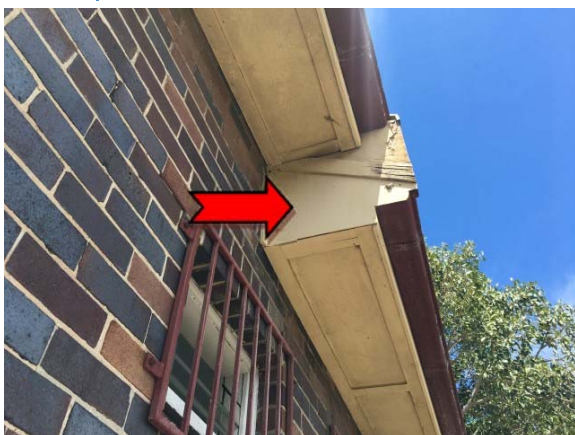
Photo 5. Exterior, ladies toilets, upstand panel – suspected asbestos-containing fibre cement sheeting.
