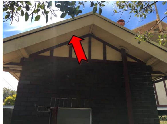
Photo 4. Exterior, ladies toilets, eaves – suspected asbestos-containing fibre cement sheeting.
