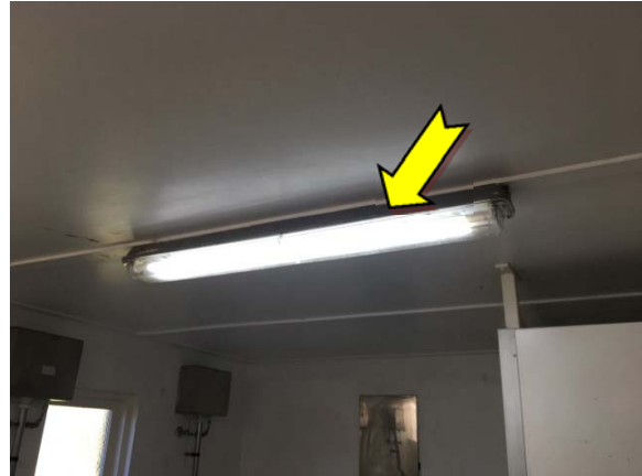
Photo 8. Interior, double tube fluorescent light fitting – suspected PCB-containing capacitor.
