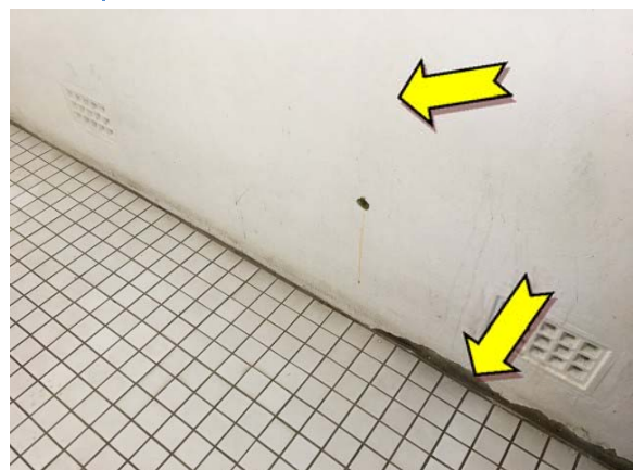
Photo 12. Interior, female toilets, walls – suspected lead-containing white upper and blue lower coloured paint systems.
