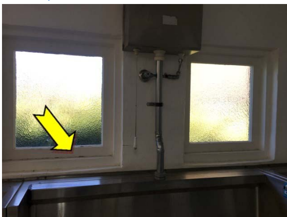
Photo 11. Interior, window frames – suspected lead-containing white upper paint systems.
