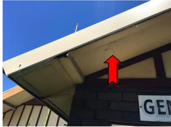
Photo 2. Exterior, male toilets, eaves – asbestos-containing fibre cement sheeting.
